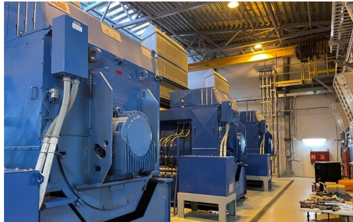
Figure 1: New Wärtsilä generation units at the Randolph Harley Power Plant, St. Thomas, USVI.
