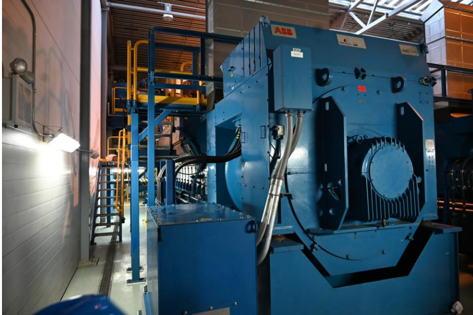
Phase I Wartsila unit at the Randolph Harley Power Plant in St. Thomas, U.S. Virgin Islands (Photo by Barry Leerdam)
