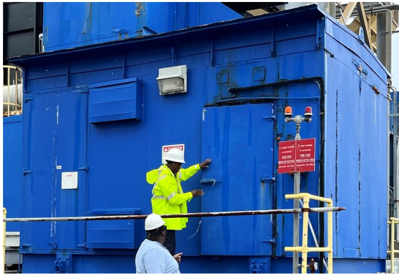
Image: WAPA Plant Personnel in front of GT20 at the Richmond Power Plant on St. Croix.
