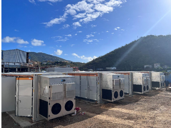
Figure 1: Multiple Battery Energy Storage Systems (BESS) on site at the Randolph Harley Power Plant in St. Thomas, USVI.
