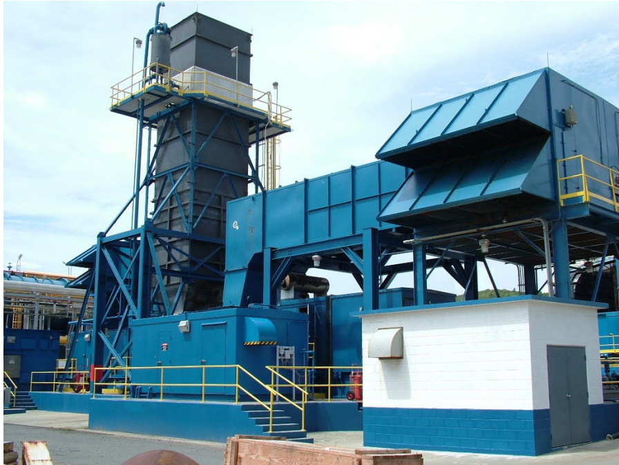
Figure 1: Virgin Islands Water and Authority's Estate Richmond Power Plant on St. Croix, US Virgin Islands.
