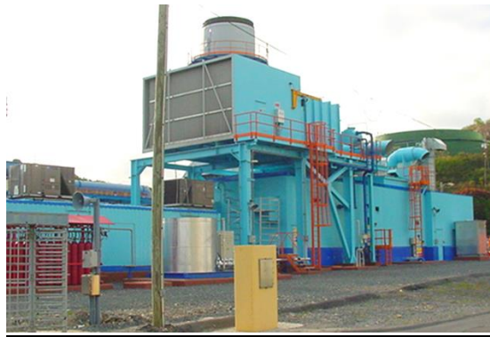
Image: Unit 23 at the Randolph Harley power plant on St. Thomas
