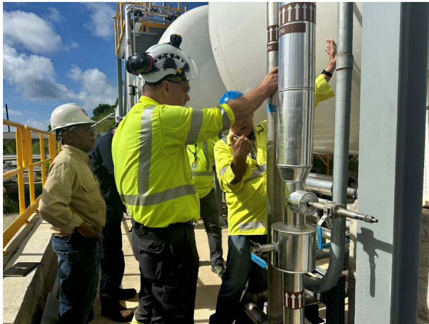
Image: Representatives from WAPA, Wärtsilä, and West Peak Energy conducting walk-through at the Randolph Harley Power Plant since remobilizing on July 15, 2024.
