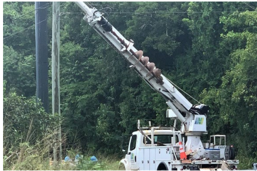
Image: WAPA Line crew and contractor, Haugland VI, working on composite pole installations.
