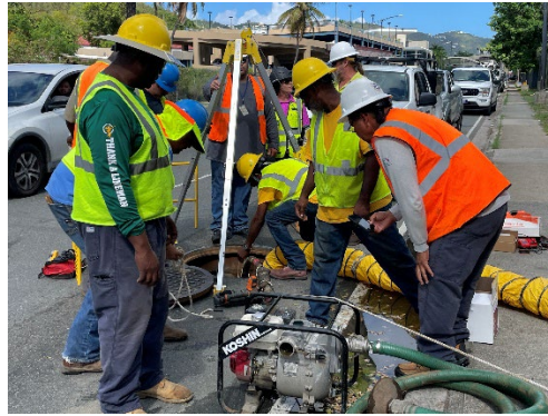
Figure 1: WAPA personnel on site troubleshooting and removing damaged cable out of manhole, as part of repairs to Feeder 13.
