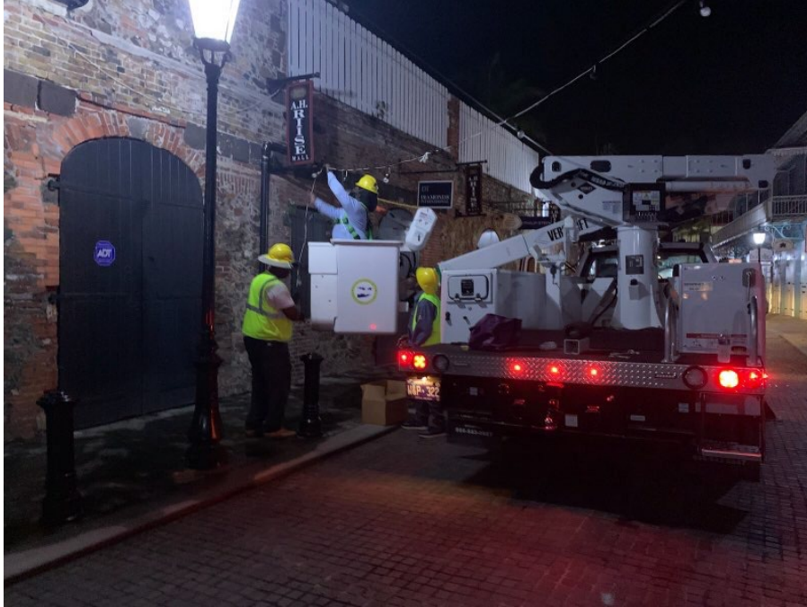
Figure 1: WAPA lineworkers use new Versalift bucket trucks to install lights for Miracle on Main Street on Tuesday, December 6, 2022. The hybrid bucket truck was funded by the Department of Interior which boasts high efficiency amongst other benefits.
