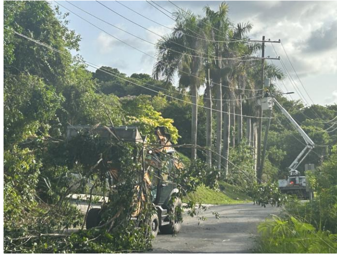
Image: WAPA Crews working on clearing debris and repairing poles in the field.
